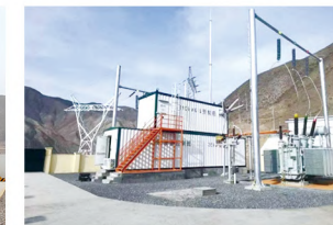
110kV Xiahe Prefabricated Substation
