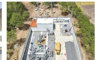
35kV Shitou Transmission & Transformation Project, China Southern Power Grid
