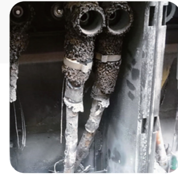
Cable connector failure
