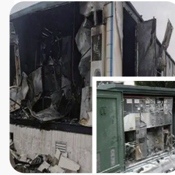
Switchgear fire accident
